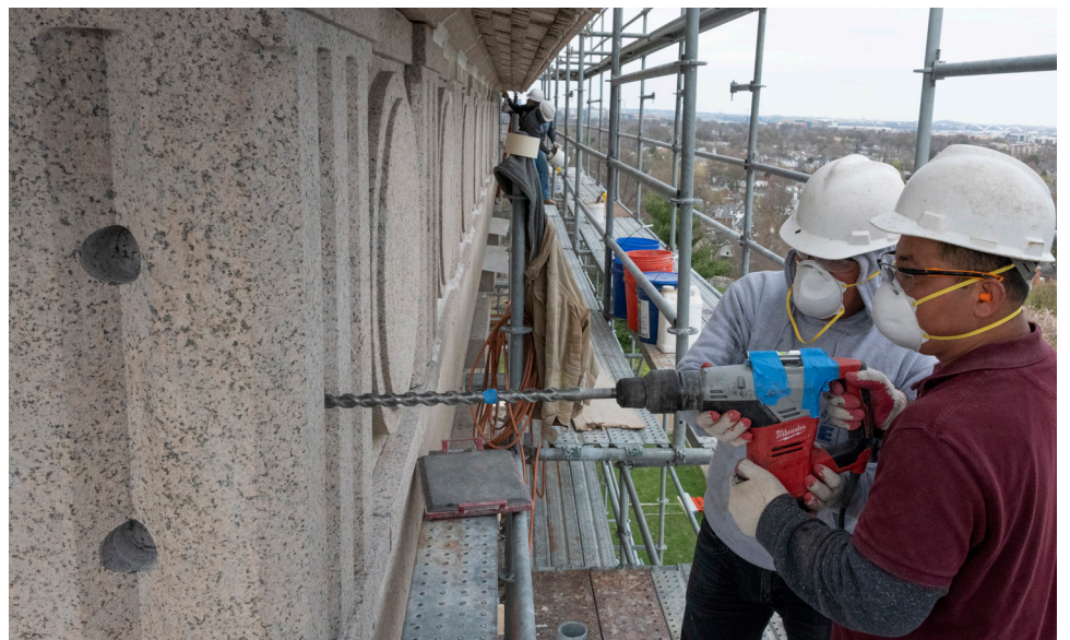
Three-foot steel reinforcements were embedded within the frieze to stabilize the corners of the entablature.
