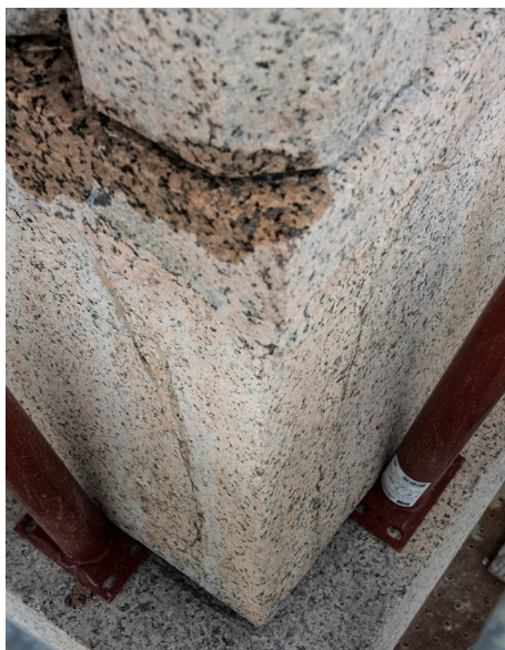
Stress fractures were visible in the corners of the architrave.
